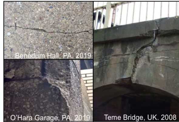
Figure 1: Photographs illustrating examples of cracked concrete.
