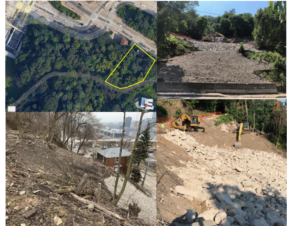
This landslide measures ~140-ft in length and ~60-ft in width
