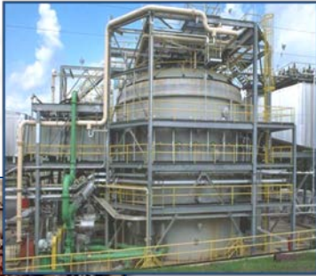
Flue Gas Desulfurization (FGD) Scrubbers
