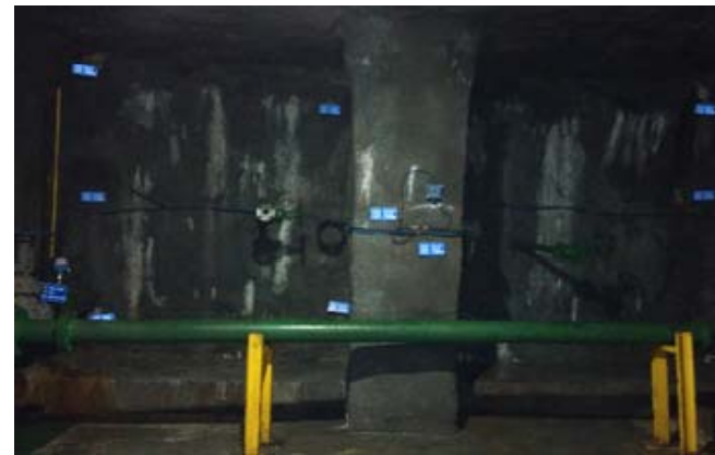
Monitoring device for the dam
