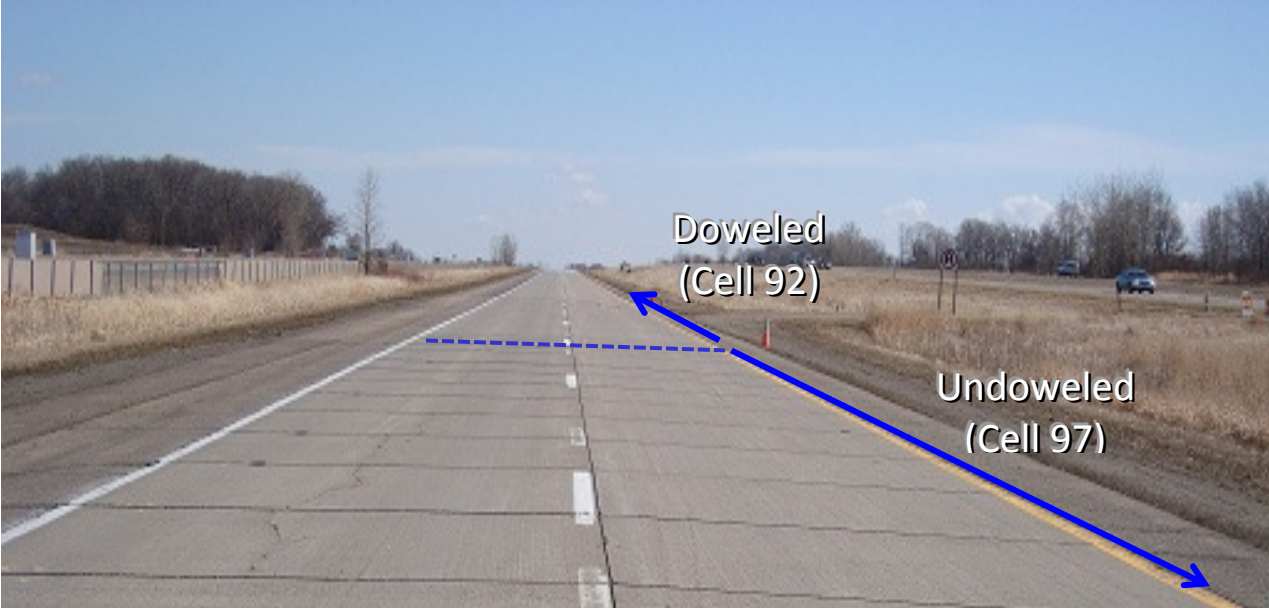
FIGURE 9 Visible faulting for the undoweled Cell 97.
