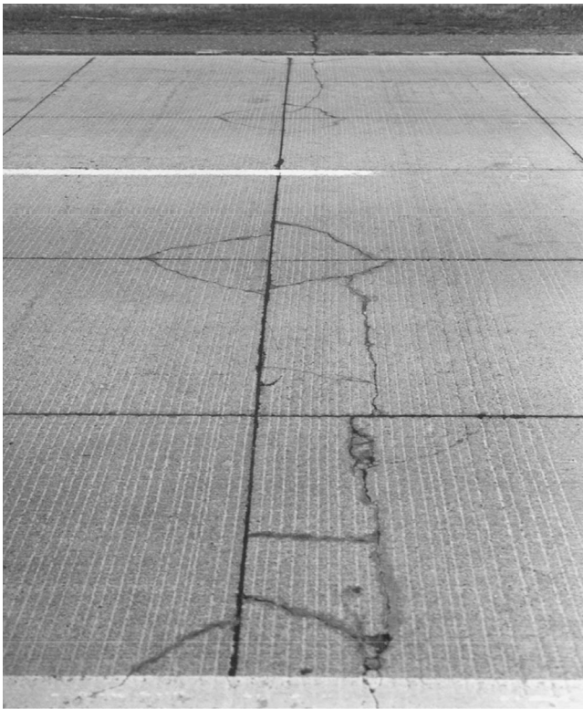
FIGURE 3 Reflective cracking in ultrathin whitetopping.
