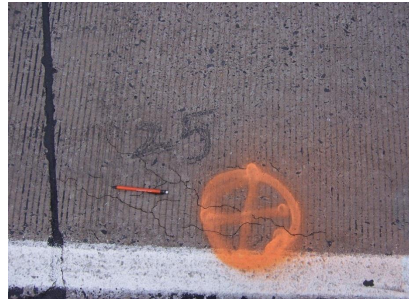
(Cracks have been digitally enhanced)
