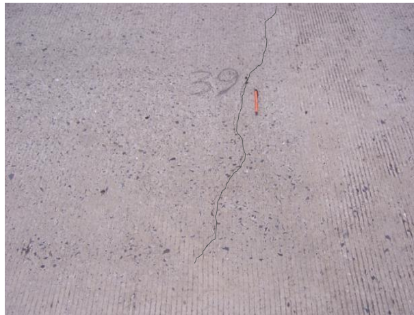
(Crack has been digitally enhanced)
