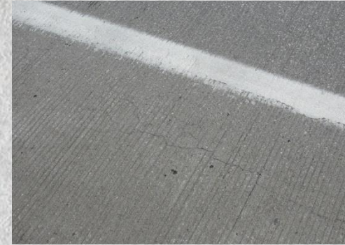
↑ hairline cracking of LMC
