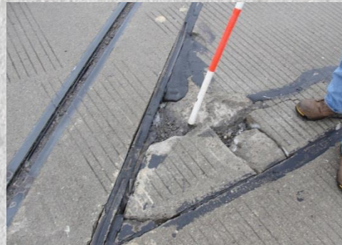
← damage near acute skew
