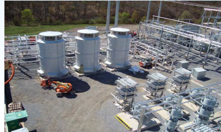
SVC – rating -100 to +250 Mvar at 230 kV
