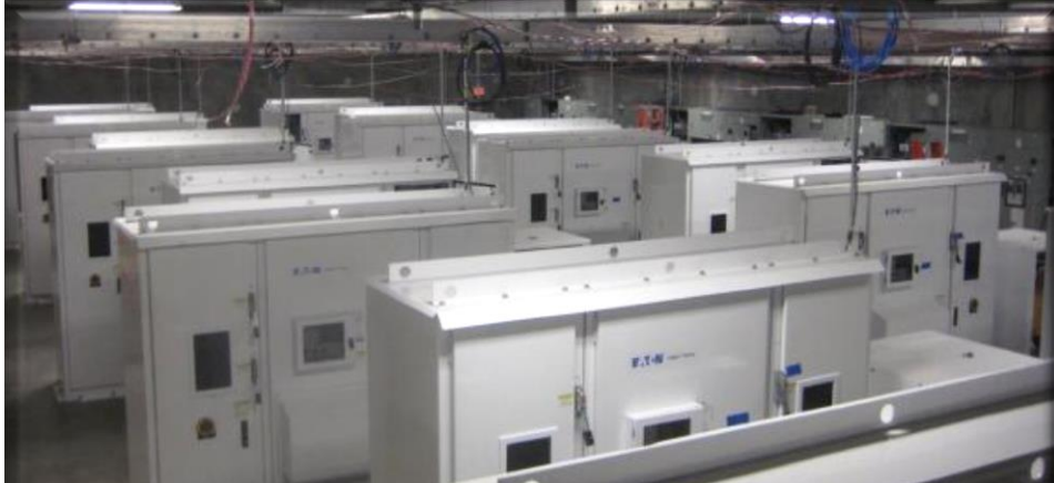
5MW Inverter System
