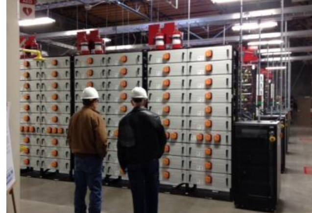
5MW Li-ion Batteries
