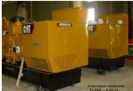
Natural Gas Generators
