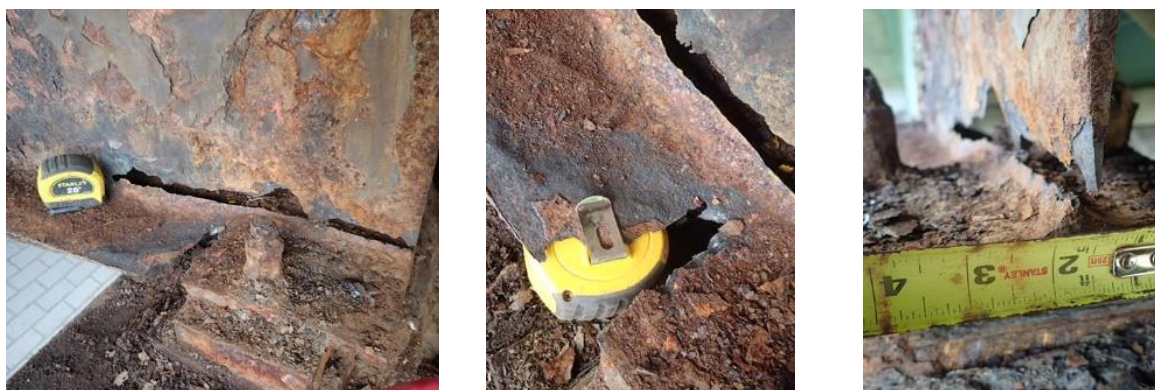
a) Pattern M1 damage (b = 17 in.; a = 1.5 in.)
