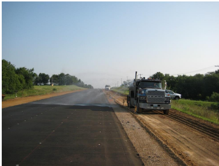
Figure 13. Misting interlayer prior to paving the unbonded overlay. (Photo courtesy of John Donahue of the Missouri Department of Transportation.)
