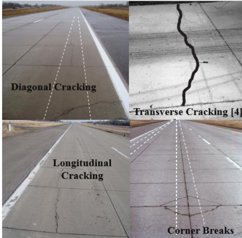
Figure 1. BCOA load-related distresses. (Transverse crack has been digitally enhanced.)
