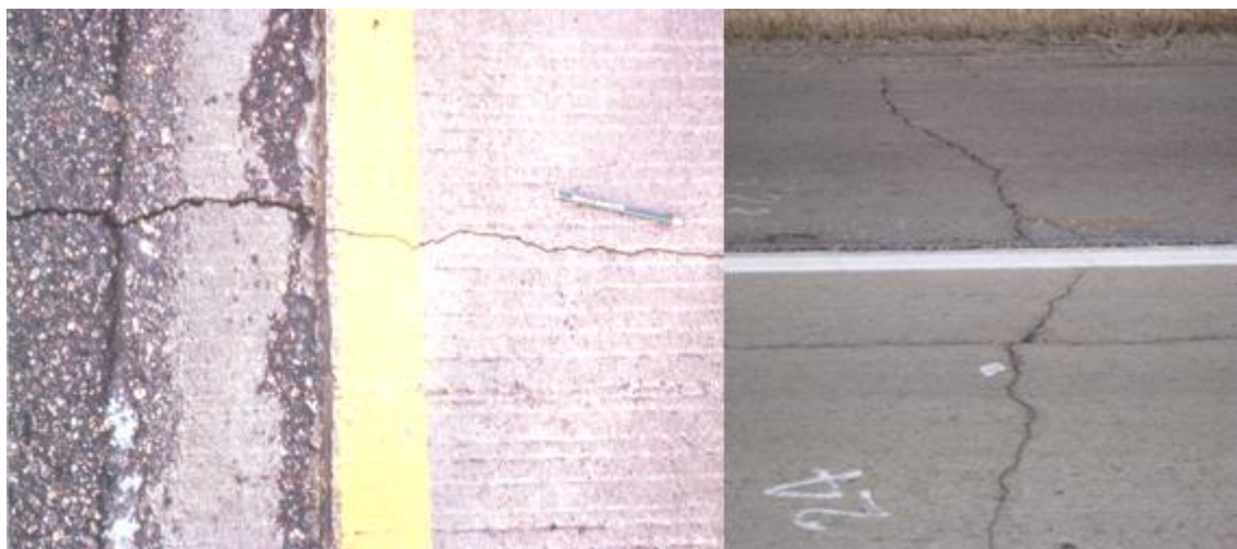
Figure 2. Reflective cracking in a BCOA.
