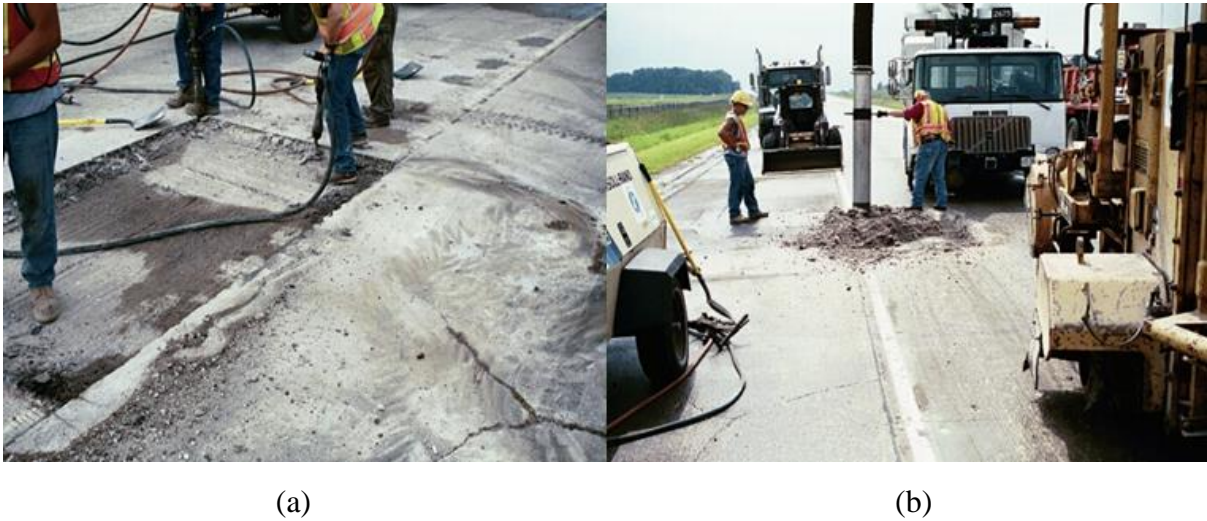
Figure 5. Material removal a.) jackhammering and removing the exterior edge and b.) removal of debris from the repair area.
