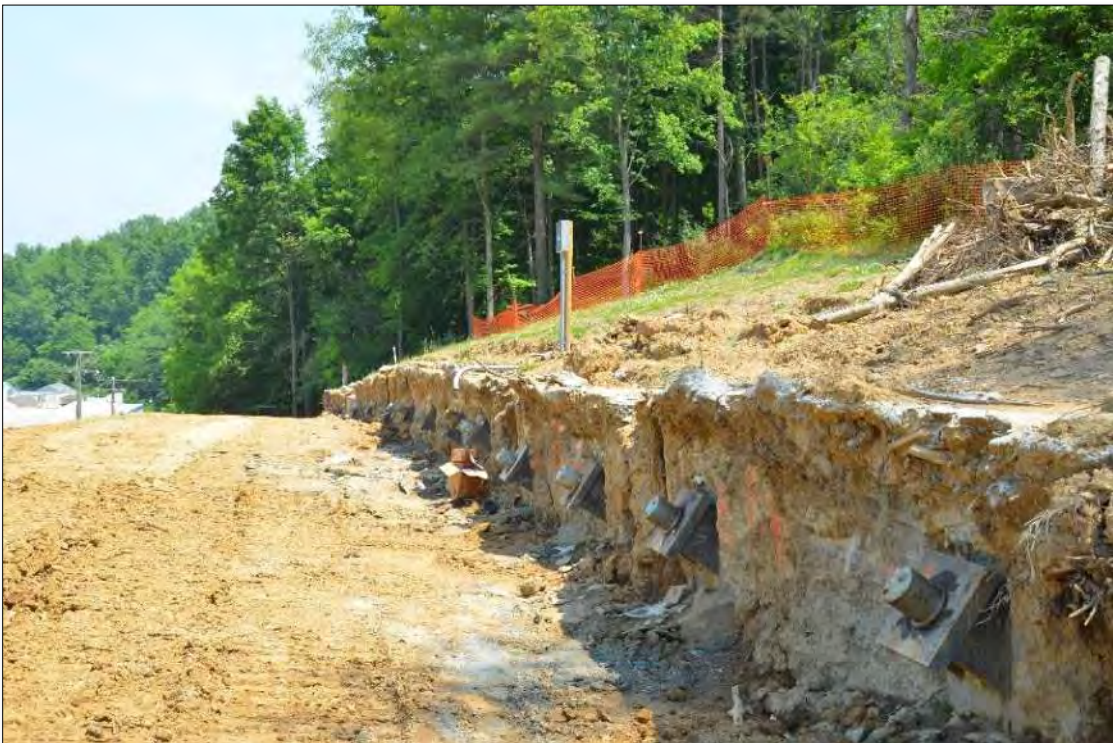
Figure 10-71 - Example Buried Panel Wall with Tiebacks, Anchors Tested, Stressed, Locked Off, and Capped
