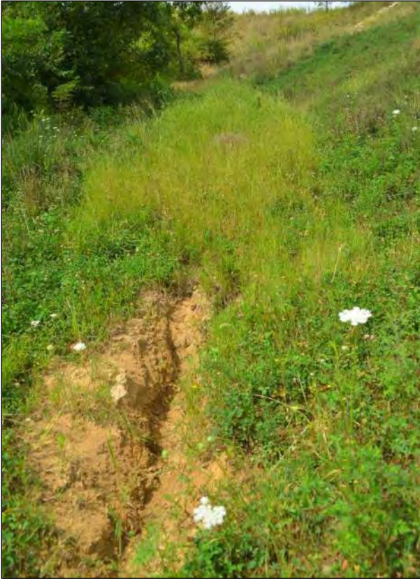
Photograph 2. Embankment Toe, Erosion Rill Looking West
