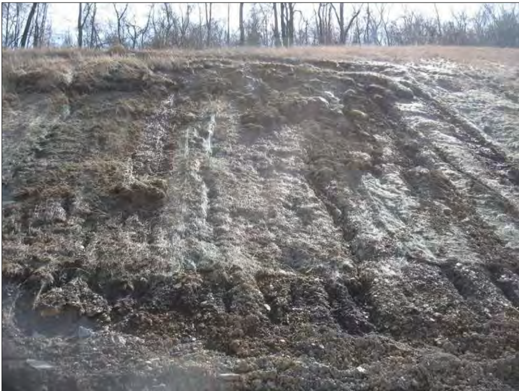
Figure 10-97 - Seepage and erosion gullies formed on the slope below the head scarp
