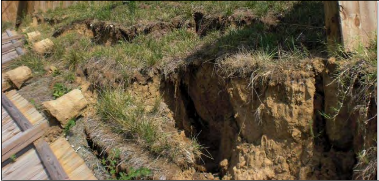
Figure 10-25 - Close-Up View of 4+ Foot Deep Erosion Rivulets Near the Ground Surface
