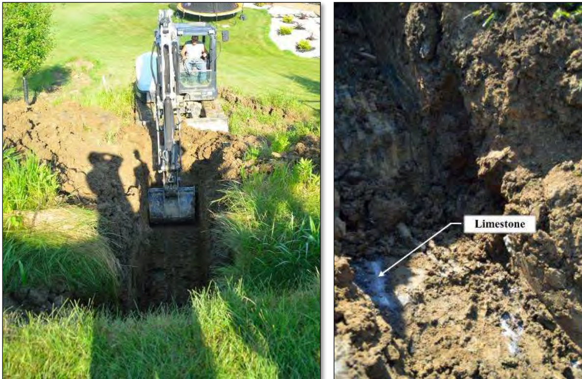
Figure 4-8 - Test pit investigation performed to confirm presence of limestone bed and wet clay soils at toe of slope identified in the desktop study; bag samples were collected for laboratory testing
