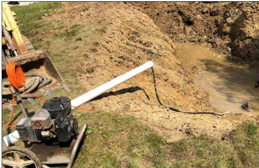
Figure 4-1 – Mitigation effort for a rotational slide caused by excess pore water pressure at the toe of slope; toe key elevation, as shown, intercepted the water bearing Uniontown limestone member
