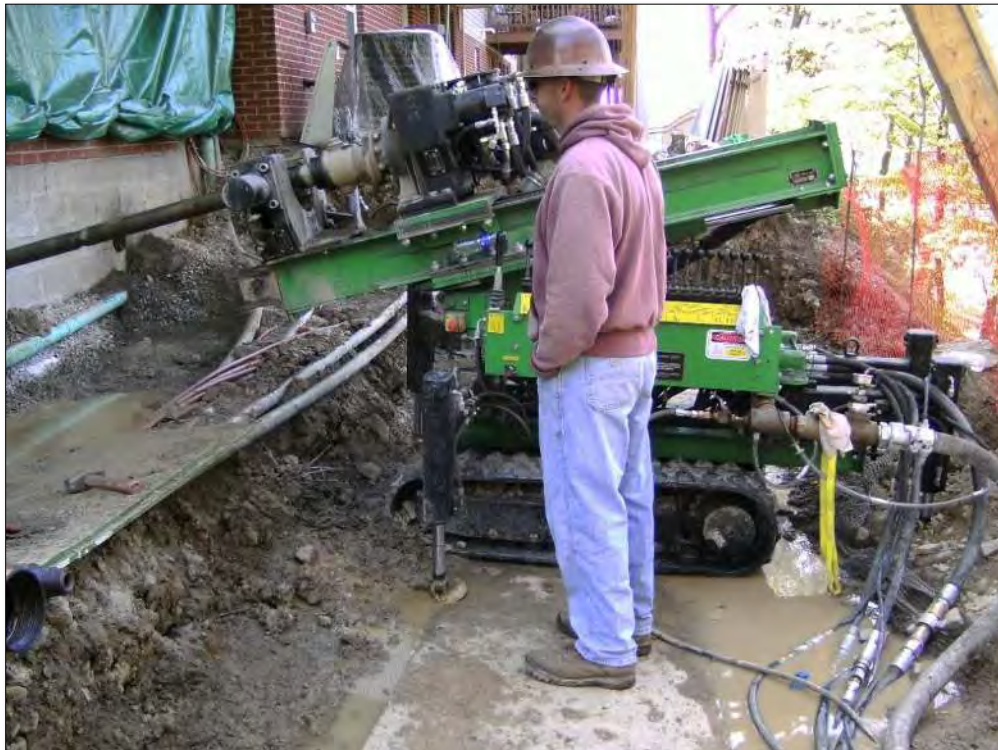
Figure 10-61 - Example Tieback Installation with a Small Duplex Drill on Top of an Existing MSE Wall, Allegheny County
