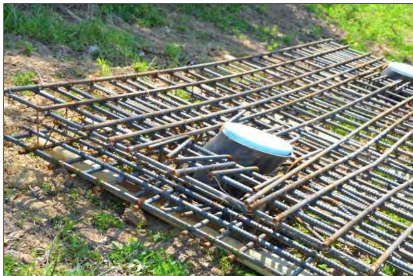
Figure 10-67 - Example Buried Panel Wall with Tiebacks, Rebar Cage with Anchor Sleeve, and Styrofoam Blockout
