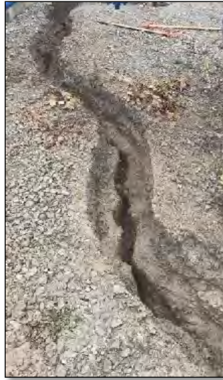
Photograph 1. Observed Tension Crack
