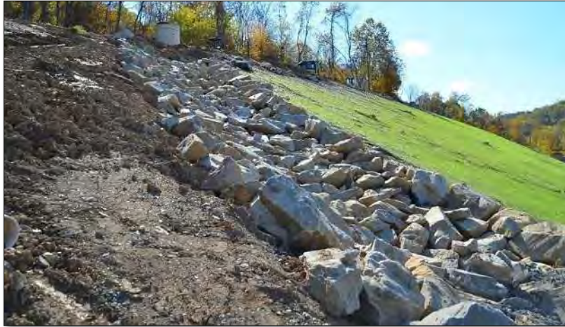
Figure 10-89 - Rock Lined Ditch
