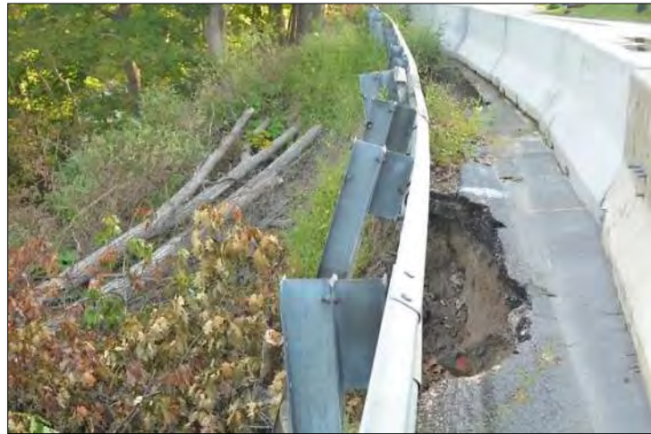
Figure 10-55 - Landslide at edge of shoulder
