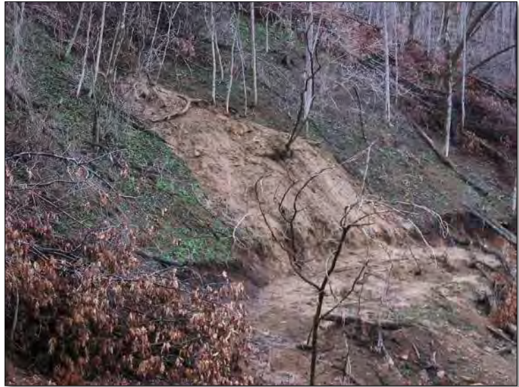
Figure 10-86 - Concentrated Overland Flow, Leading to an Eventual Landslide, Fayette County, PA
