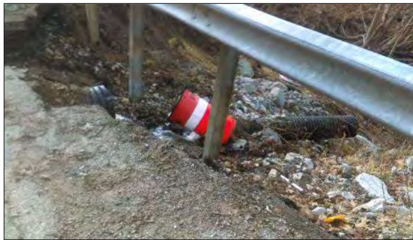
Figure 8-4 - Separated underdrain causing excessive slope erosion leading to a landslide which comprised the shoulder of a roadway (PennDOT District 11)
