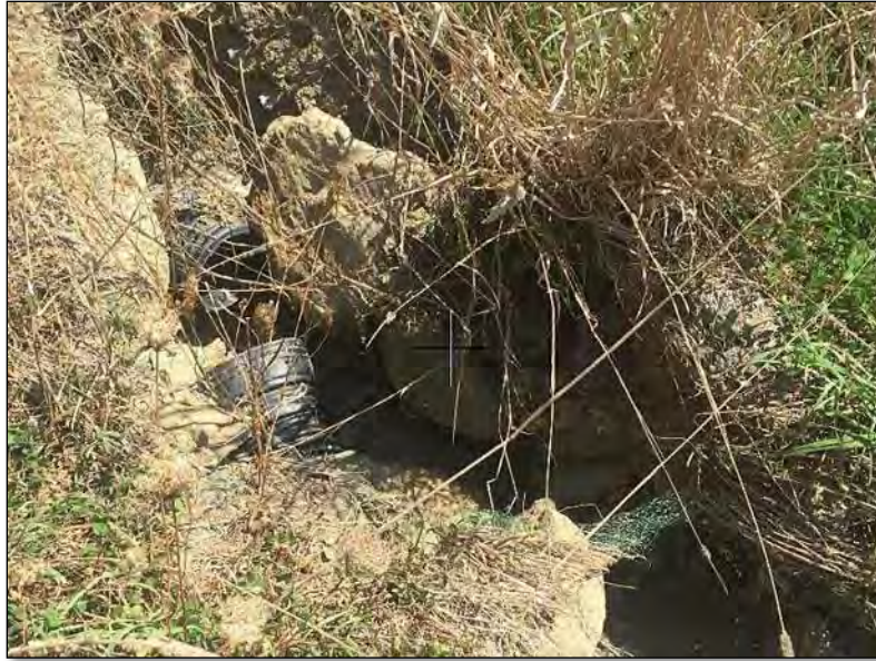
Figure 8-3 - Separated subsurface drainage pipe leading to erosion of the subgrade
