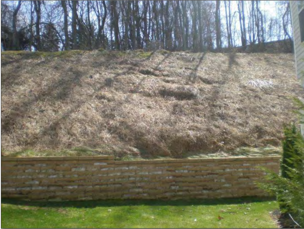
Figure 10-21 - Shallow slope failure
