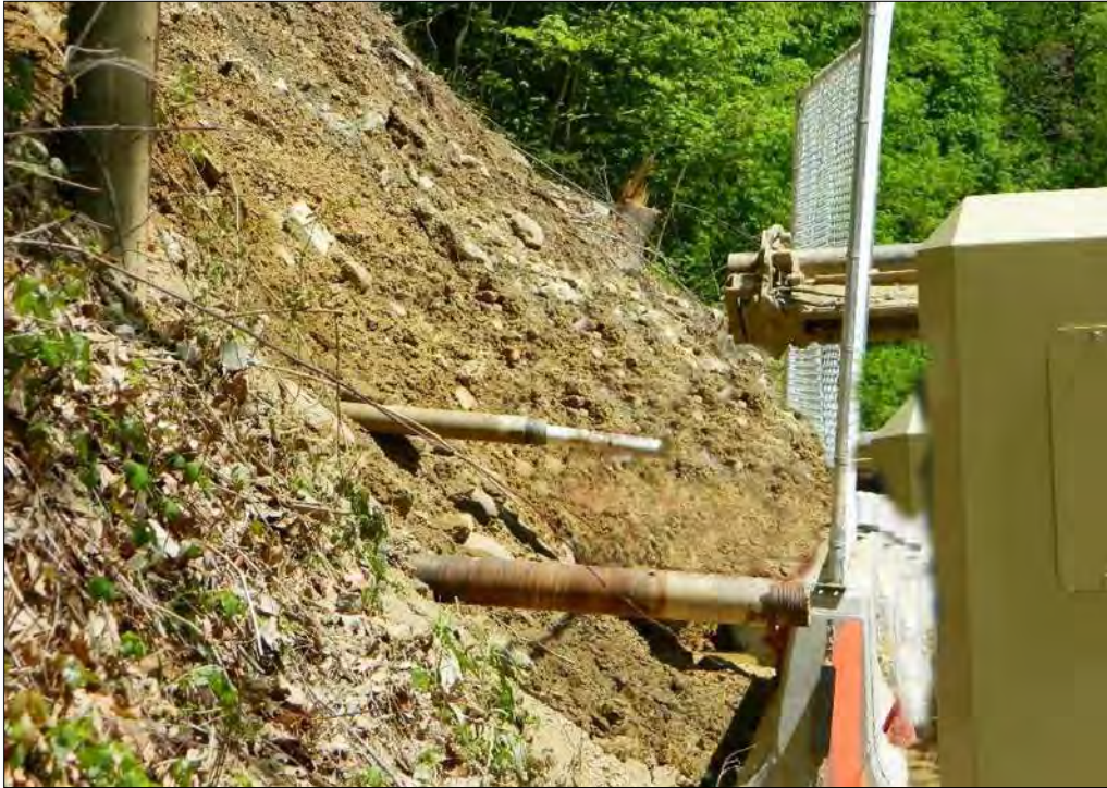
Figure 10-103 - Slotted Well Screen and PVC Conveyance Pipe Through Surface Casing to Install Horizontal Drains
