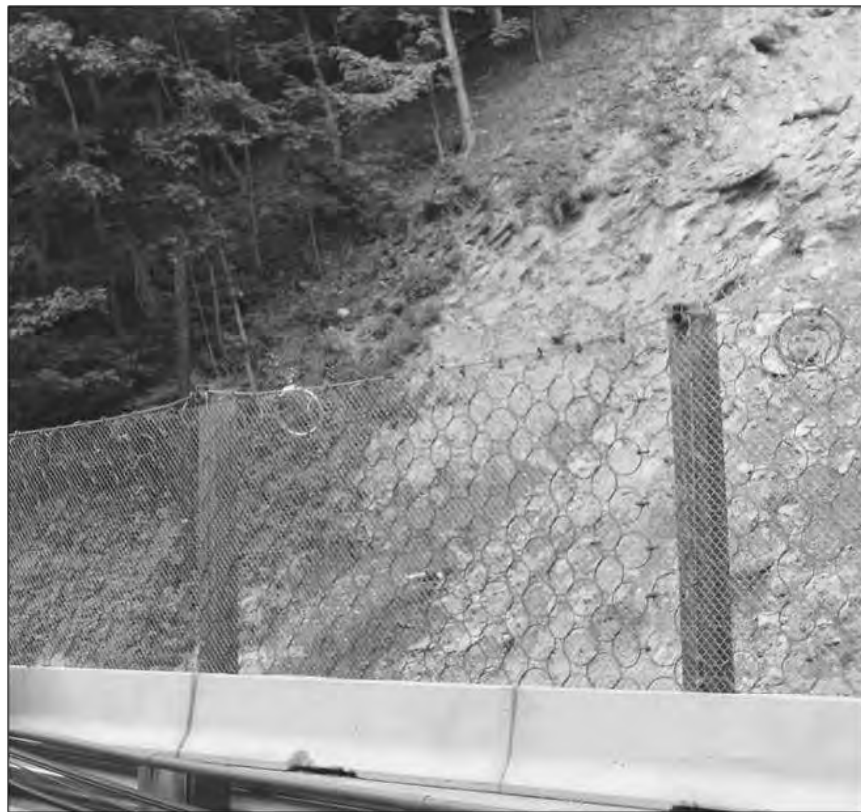
Figure 10-116 - Debris Flow Fence
