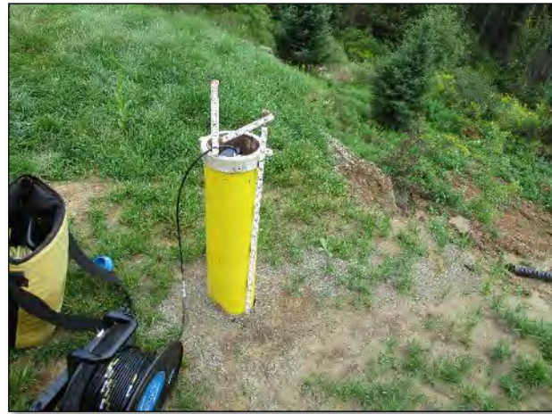
Figure 6-11 - Inclinometer Reading at Crown of Landslide
