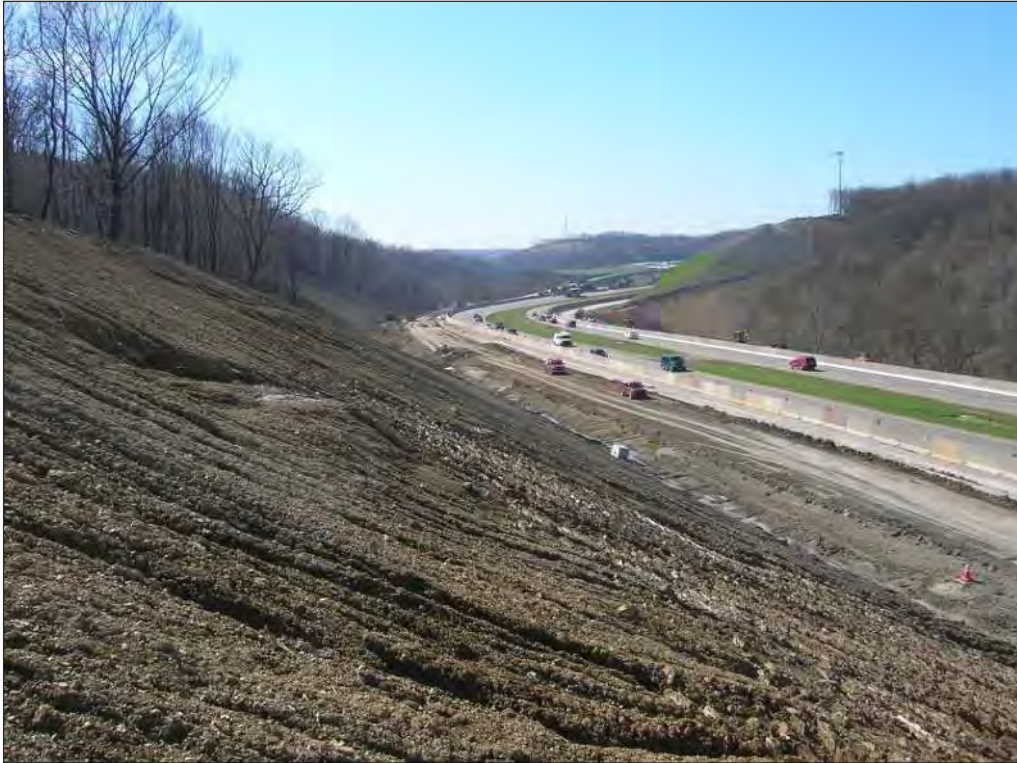
Figure 10-98 - Slope cleared to allow for identification of seepage points and installation of finger drains
