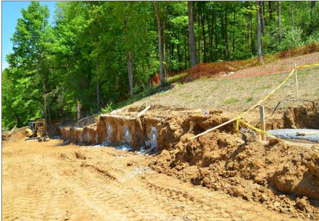
Figure 10-69 - Example Buried Panel Wall with Tiebacks, Front Face of Panel Partially Exposed
