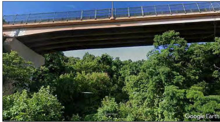
Figure 10-4 - “Bridging” Example Aerial View of McArdle Roadway Spanning over Landslide, Pittsburgh, PA [60]
