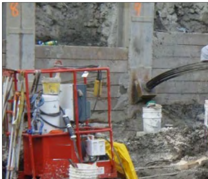
Figure 10-65 - Example Tieback Wall with Timber Lagging and Multistrand Anchors, Allegheny County, PA
