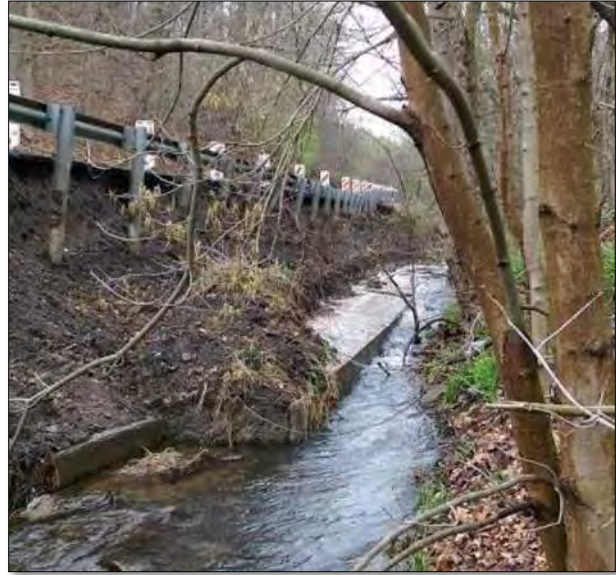
Figure 10-47 - Slope Failure along Stream Bed in Washington County, PA (PennDOT District 11)
