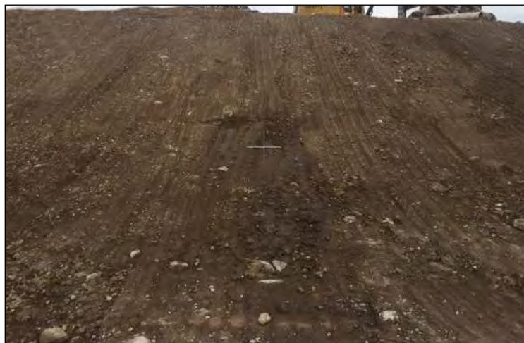
Figure 8-7 - Seepage observed on slope
