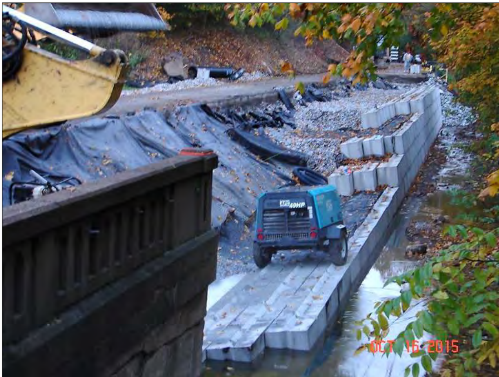
Figure 10-46 - Modular Block Wall Installed for Landslide Repair in Washington County, PA (PennDOT District 11)
