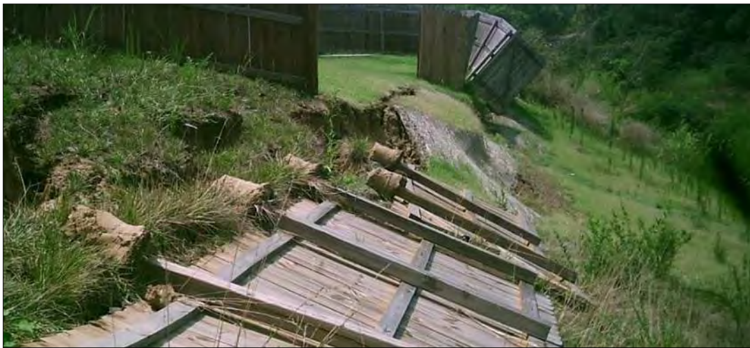
Figure 10-24 - Erosion Gullies in Loamy Soil
