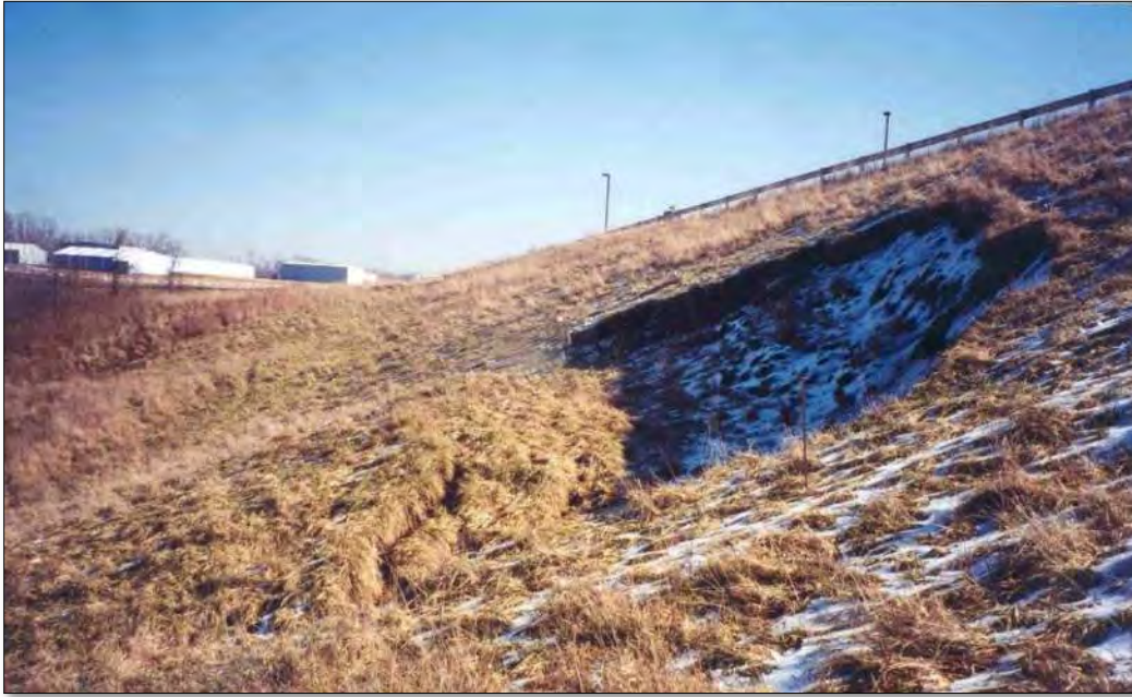
Figure 10-12 - Slope Failure (prior to mobilization of construction equipment)
