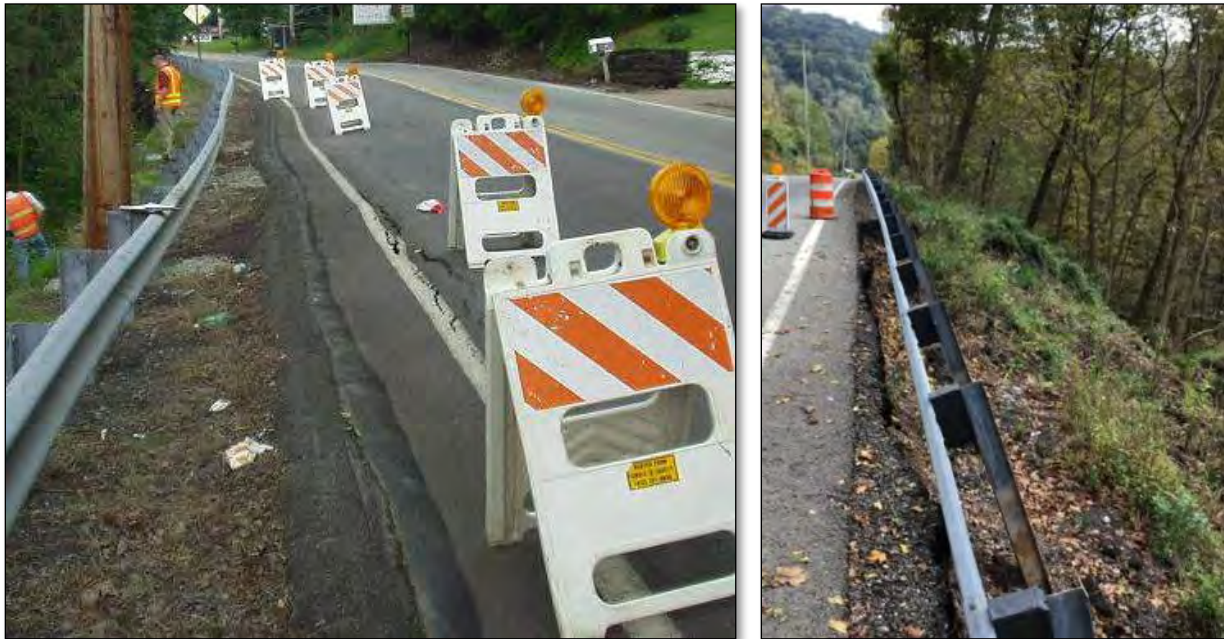
Figure 8-14 - Tension cracks on pavement observed (left), leaning guiderail (right) (PennDOT District 11)
