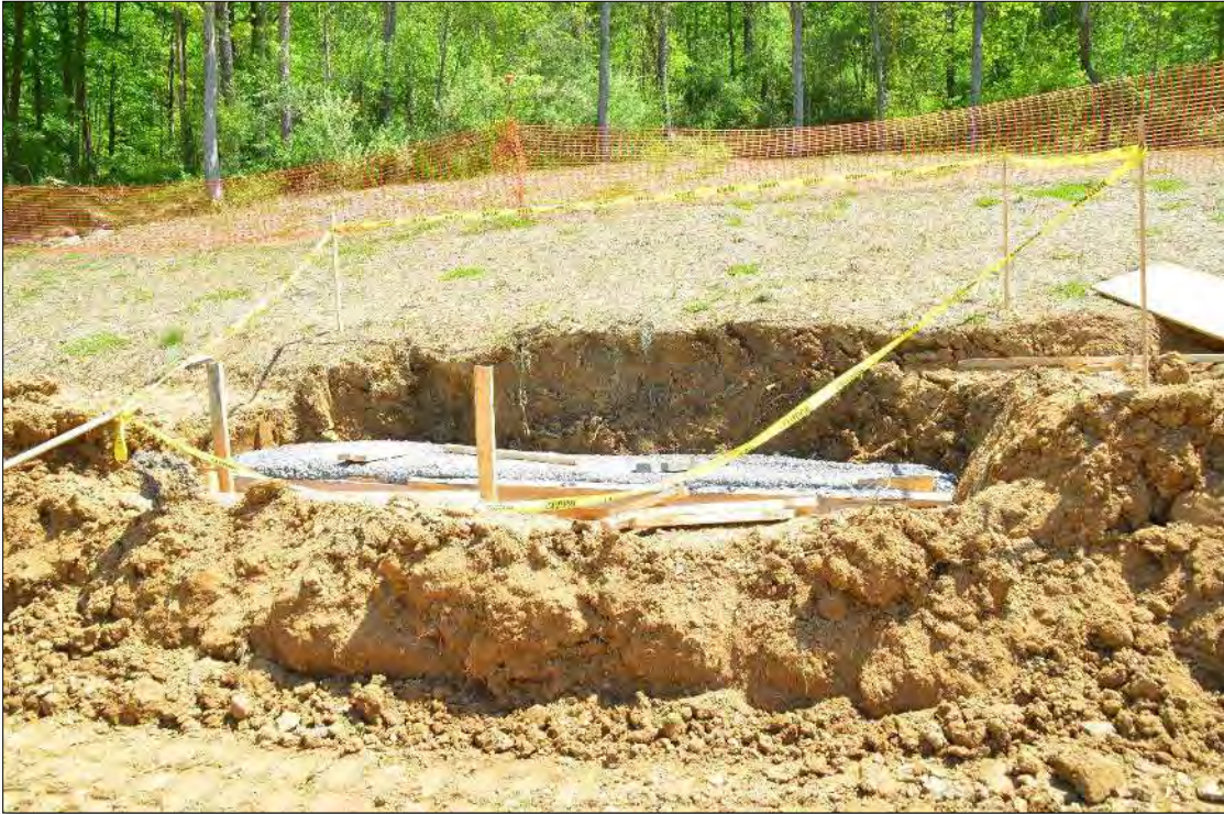
Figure 10-68 - Example Buried Panel Wall with Tiebacks, Trench After Rebar Cage is Set and Concrete is Placed Neat
