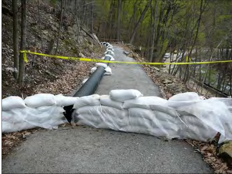
Figure 10-87 - Example of How Sandbags and HDPE Pipe Are Used to Divert Flow from an Active Landslide
