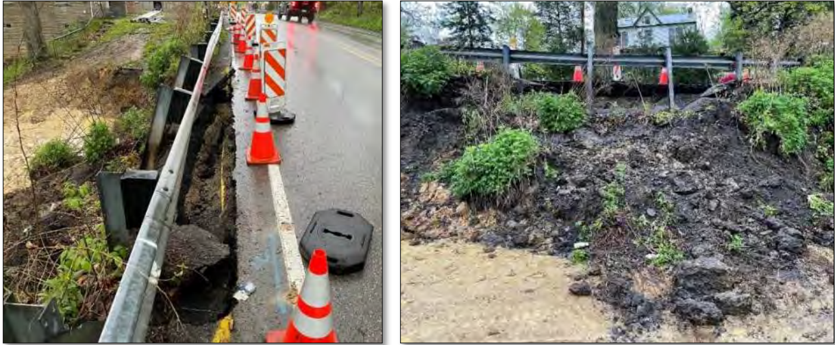
Figure 10-10 - Rock-Fill Buttress Example - Active Slope Failure Looking Down Roadway (left) and Upslope from Toe (right)
