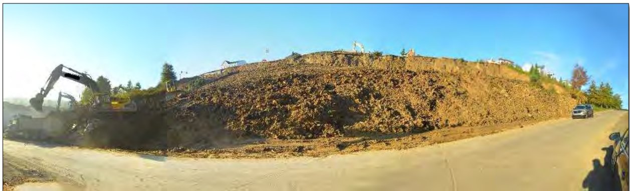
Figure 10-3 - Removal Example Massive Landslide
