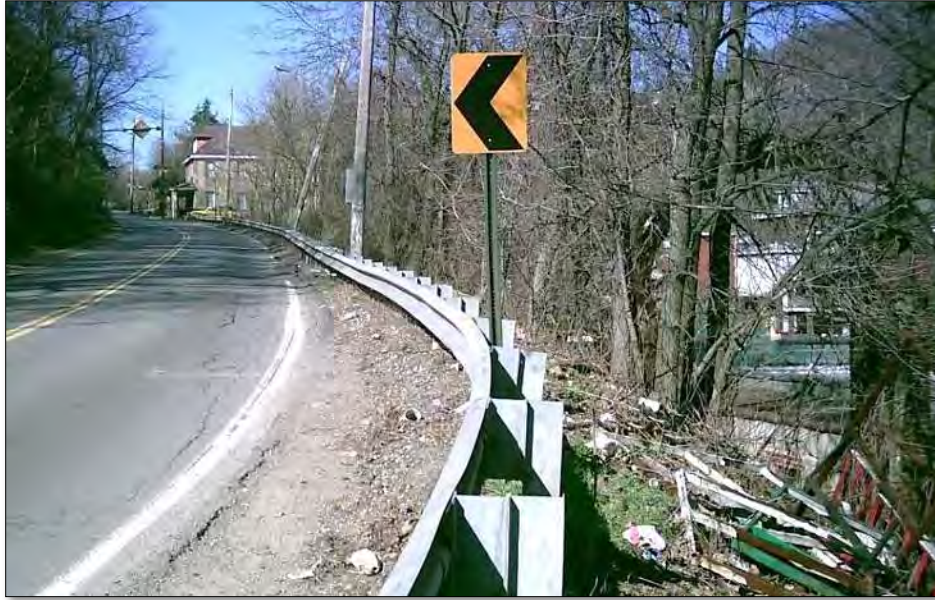
Figure 10-50 - Distressed Roadway Before Slope Repair
