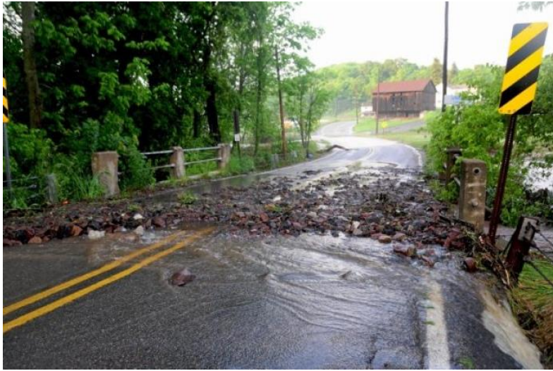
Debris on road
