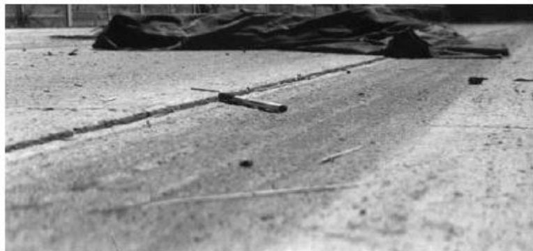
Figure 6: Typical UTW longitudinal faulting at the FHWA ALF. (Rasmussen et al., 2002)
