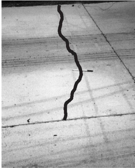
Figure 4: Typical UTW transverse cracking at the FHWA ALF. (Rasmussen et al., 2002)
