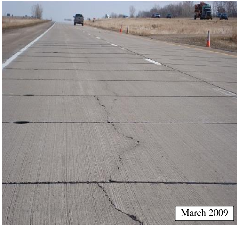
Figure 20: Longitudinal cracks in Cell 97.
