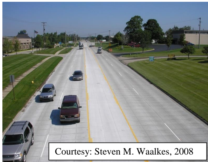
Figure 48: Condition of the UTW after two years (2008).
