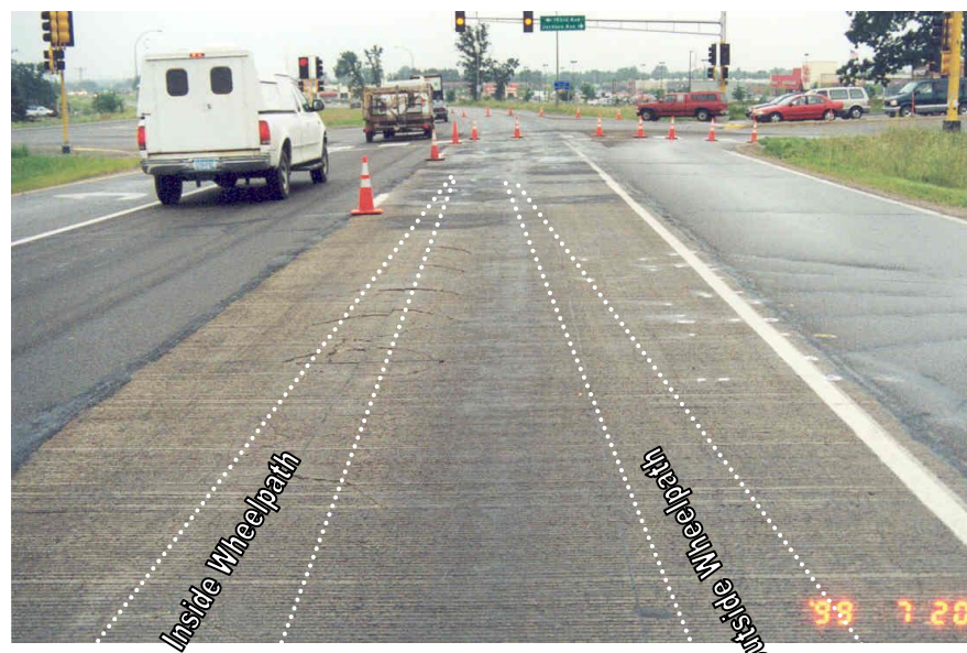
Figure 36: Corner breaks in the inside wheelpath at the Jackson Street test section. (07.20.99) (Vandenbossche, 2003)
