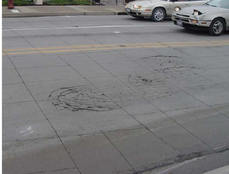
Figure 44: Distressed panels at the intersection. (Winkelman, 2005)
