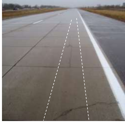
(b) Cell 63: 4in; 6ft × 5ft (March 2009)
