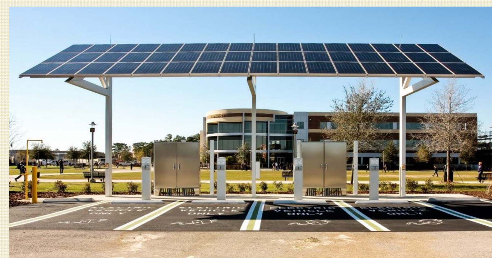
Installed Electric Vehicle Charging Station (C. S. CCJ Digital, (2011). Eaton Research Facility Adds EV Charging Stations)
