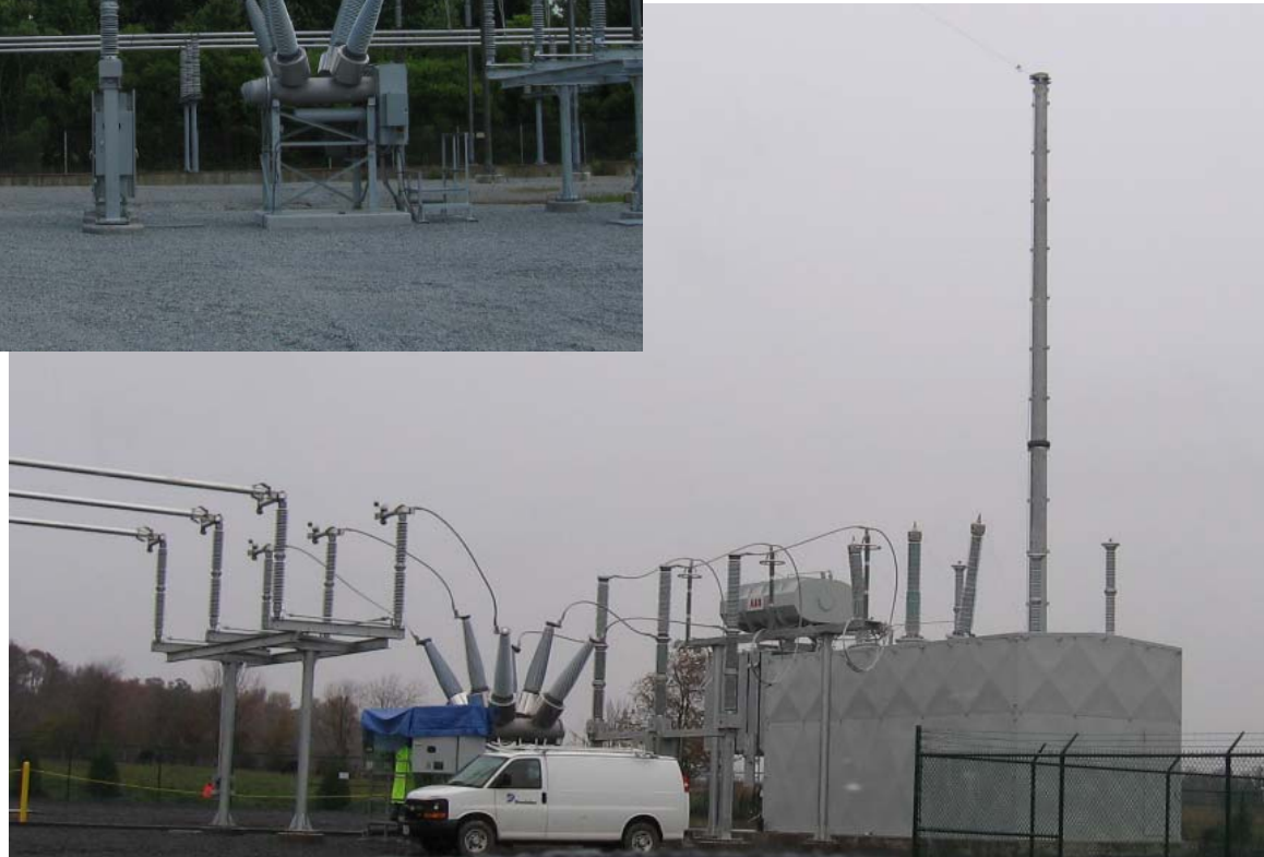
Hamilton Substation with sound enclosure
