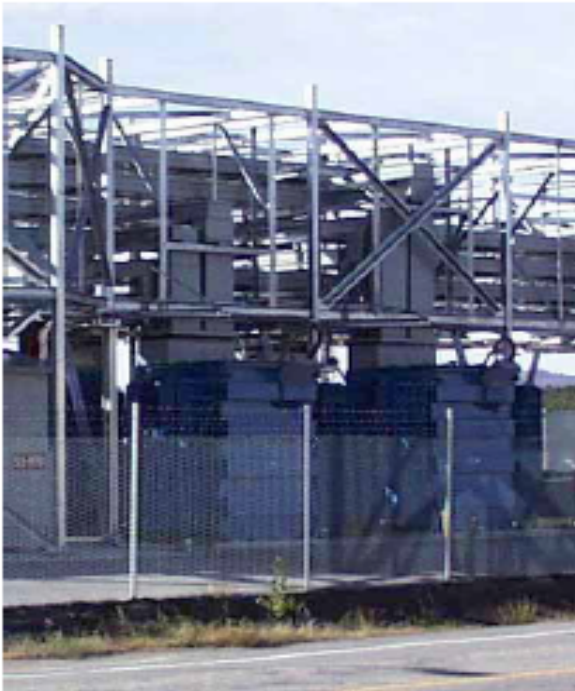
Typical H.V. Transformer
