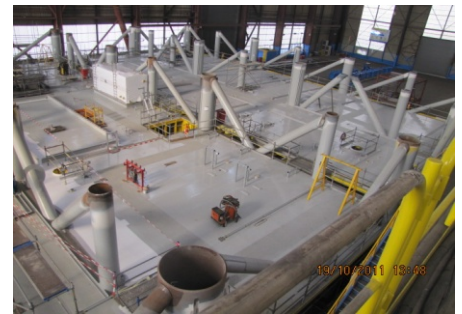
DolWin1 800 MW HVDC connection 2013
