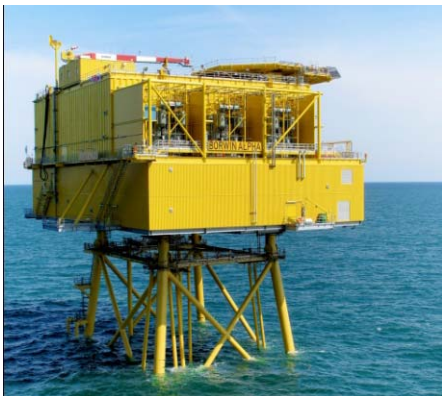
BorWin1 400 MW HVDC connection 2009
