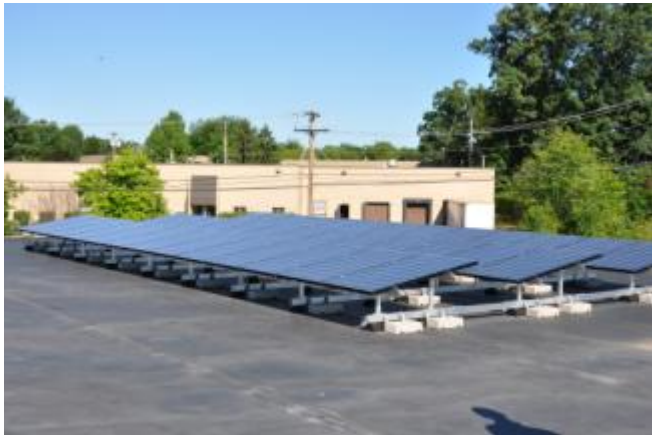
39 Panels w/Unirac mounting
