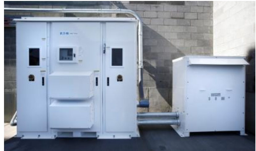
Eaton 250 kW solar inverter
