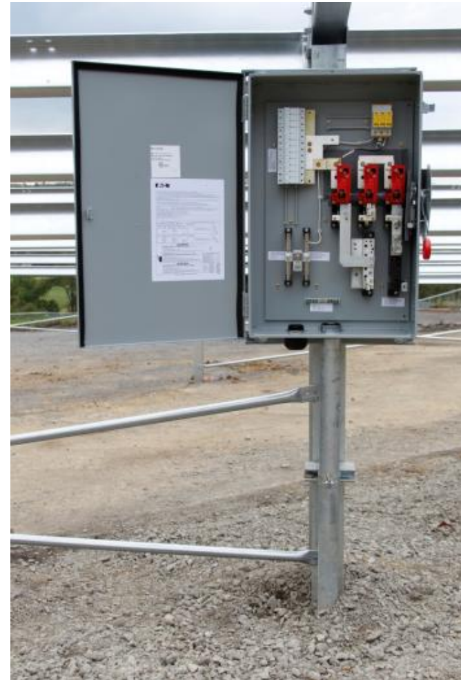
Eaton DC switch combiner
