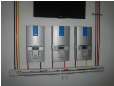
7 kW Grid-Tie Inverters
